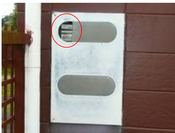
Broken meter box window
